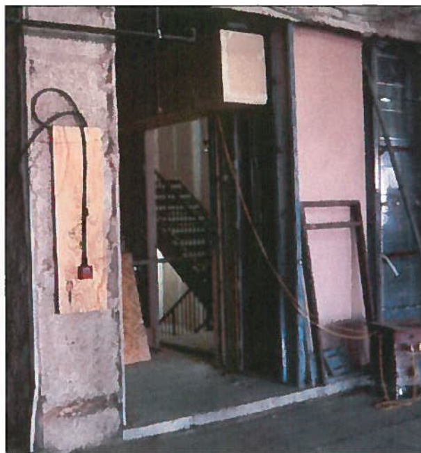
Figure 8(b) This escape route will quickly fill with smoke in a fire because no fire door is fitted
